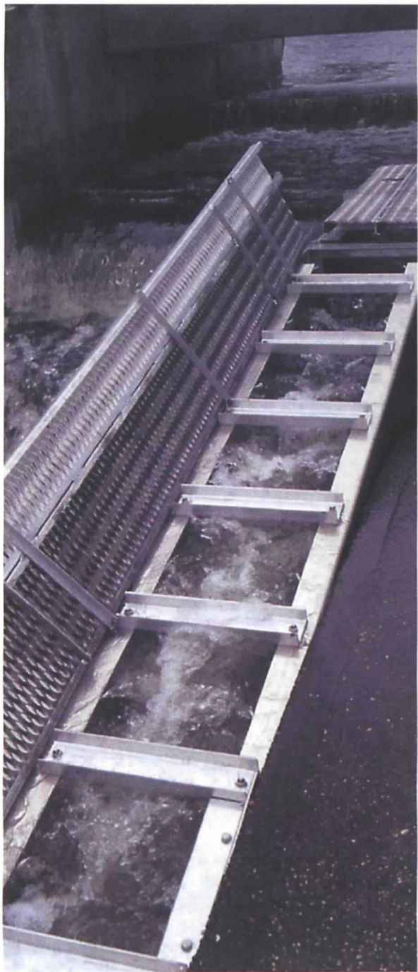
Alaskan steep pass ladder erected at the first dam on the Peconic River; it was moved eight feet to the other side of the spillway, where it proved more effective.
