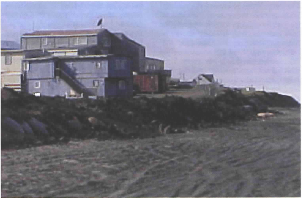
The beachfront at Barrow, Alaska. Various shore protection devices - rocks, gabions, and sand bags - have been placed at the beach's bluff to protect the town.
