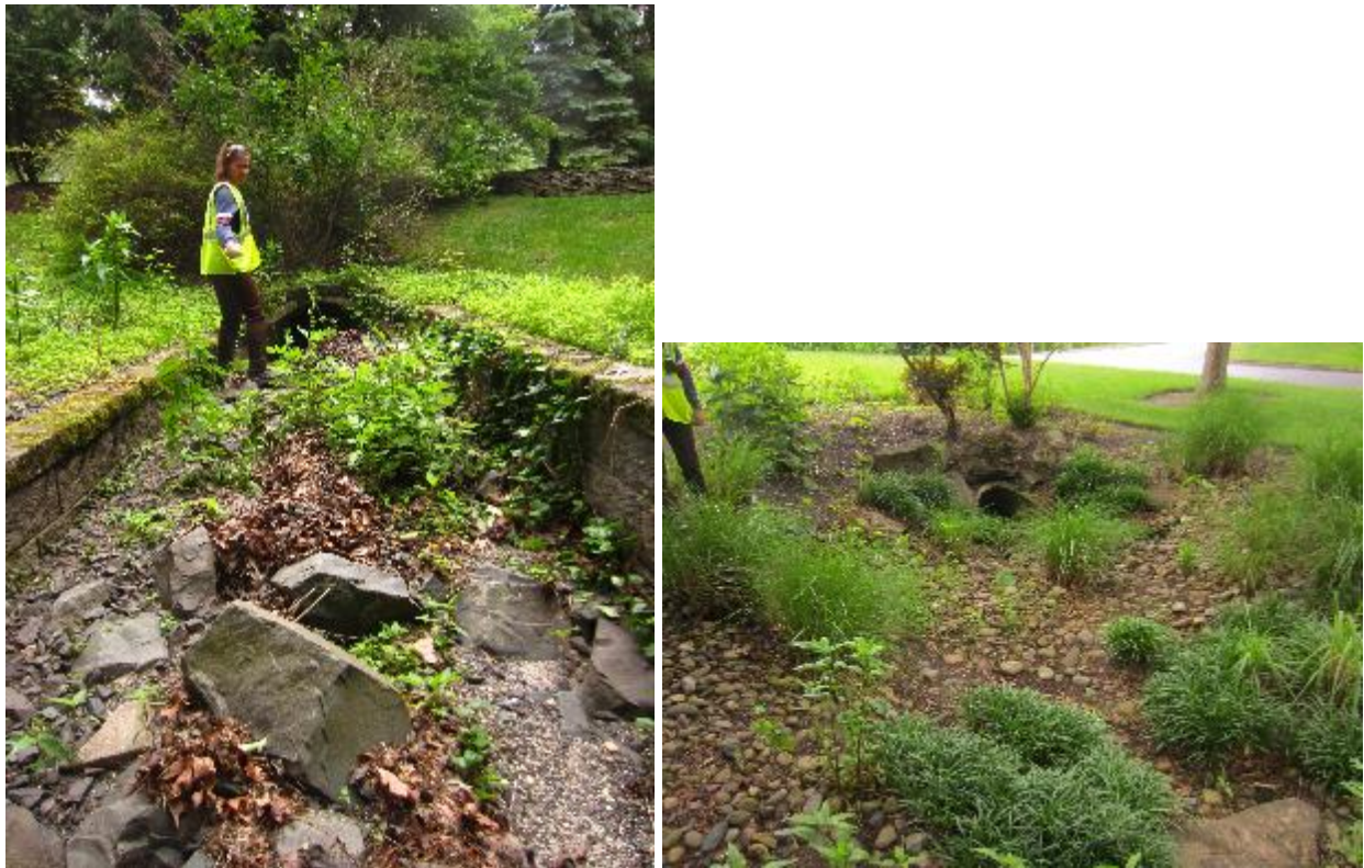
Figure 67. Culvert at Shadowbrook Dr. (downstream left photo, upstream right photo). End location for June 4, 2015 survey.
