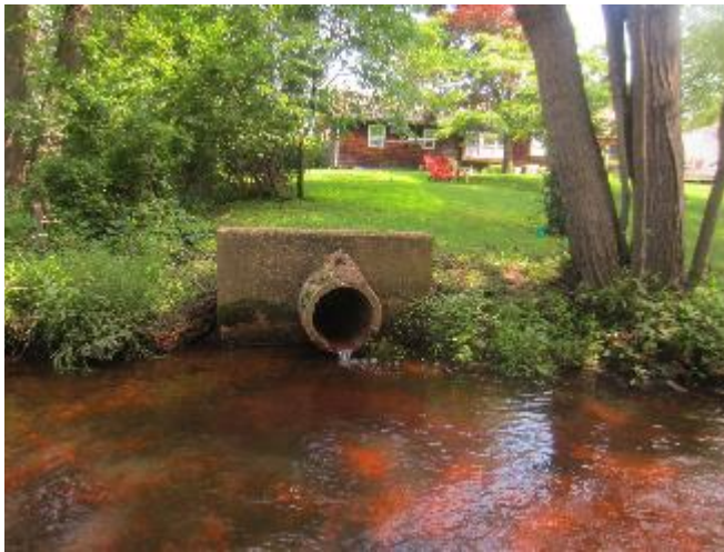
Figure 86. Culvert at the upstream end of brown, shingled house. GPS: 40.14175N 74.05025W ±21'.
