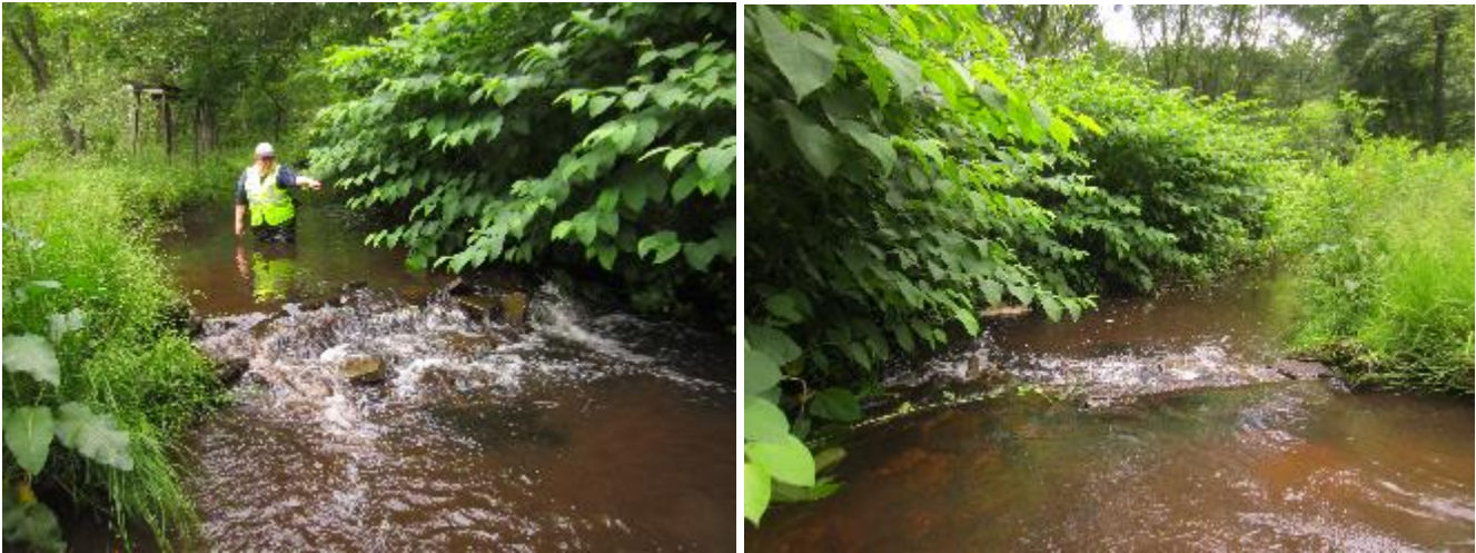
Figure 59. Small check dam located at GPS: 40.14227N 74.06844W. Looking upstream (left photo), looking downstream (right photo).
