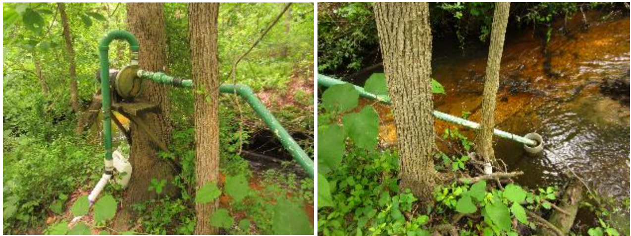
Figure 54. Pump system in-take in creek runs to house on adjacent property. GPS: 40.14161N 74.06663W \pm 30' .
