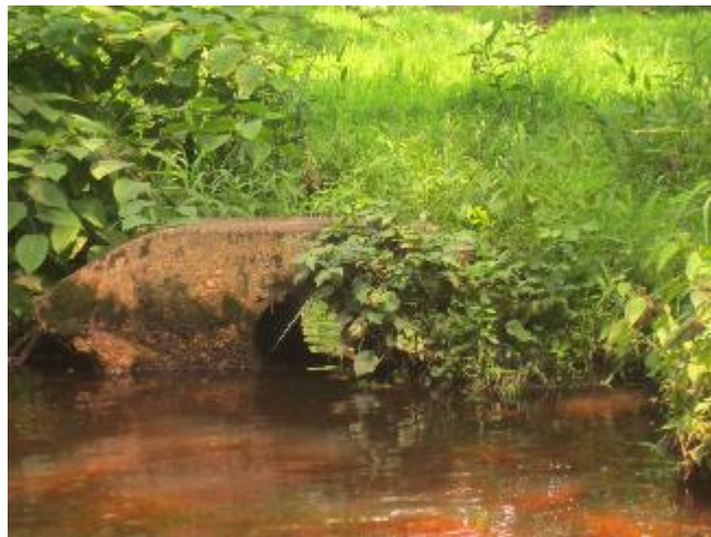
Figure 87. Culvert opening not connected to anything just upstream of culvert in Figure 86.
