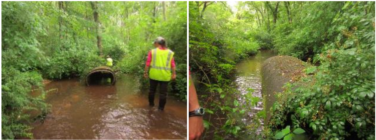
Figure 78. Large, single concrete pipe at GPS: 40.14717N 74.07893W ±36' (looking upstream left photo, downstream right photo).
