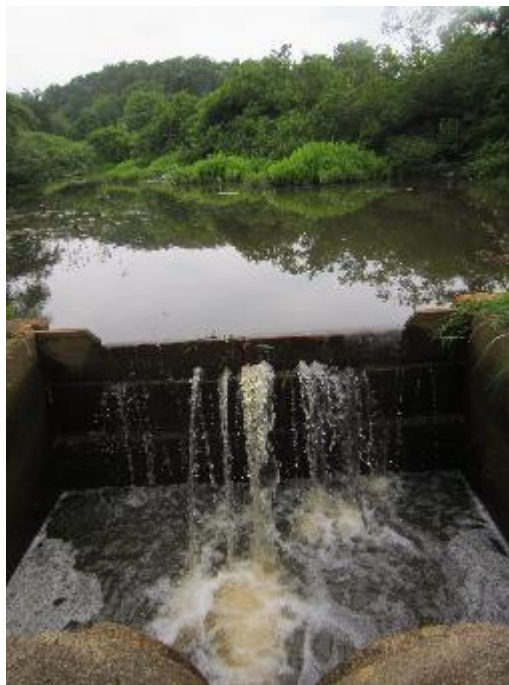
Figure 73. Broken wooden weir. GPS: 40.15263N 74.09178W ±11'.
