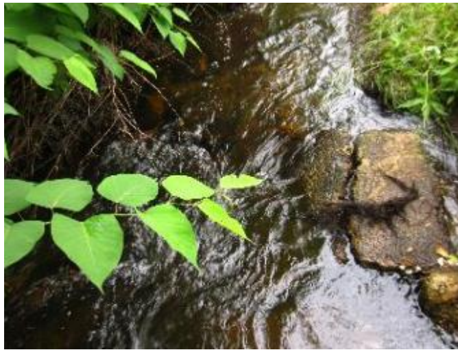
Figure 47. Small step of concrete rip rap fallen into creek from stream bank.
