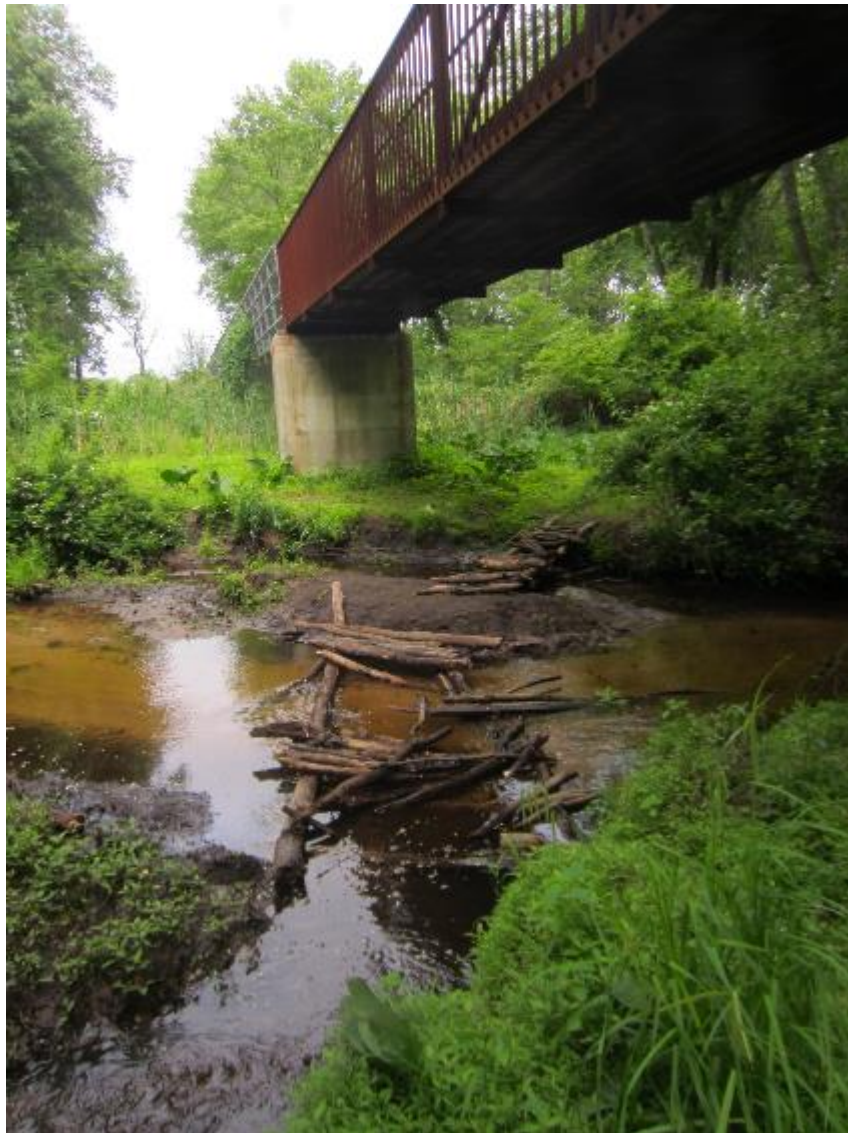
Figure 60. Hand-placed wooden foot bridge beneath bike path. Creek splits just upstream of this.
