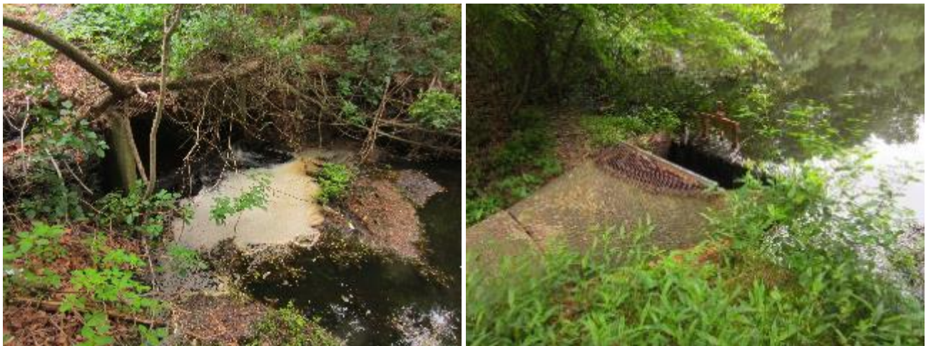
Figure 63. Culvert at downstream end of Crystalbrook Dr. (left photo) and upstream (right photo).
