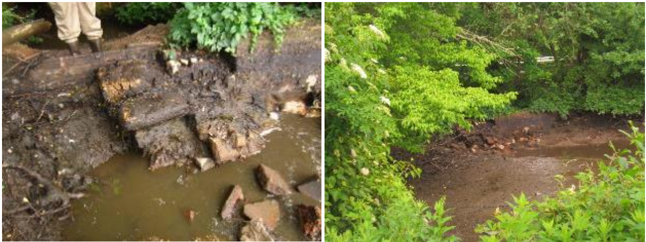
Figure 69. Broken weir upstream of Allaire Rd (downstream of mudflat in above photo).
